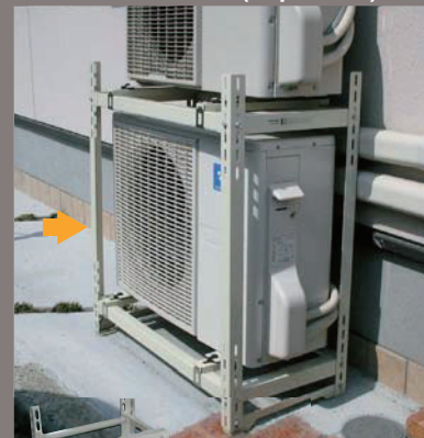
▲ Trestle for outdoor unit of air conditioner (painted)
