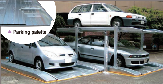
▲ Multistory mechanical parking garage
