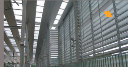
▲ Sound barrier louver (station building)
