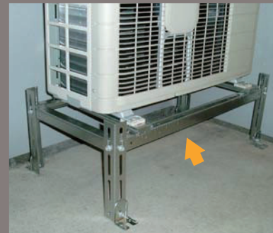
▲ Trestle for outdoor unit of air conditioner (unpainted)
