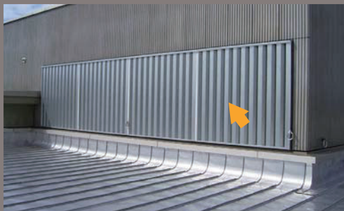
▲ Sound barrier louver
