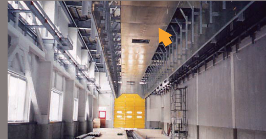
▲ Ventilation duct for train depot
