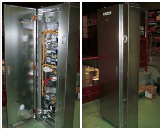
▲ Power control board
